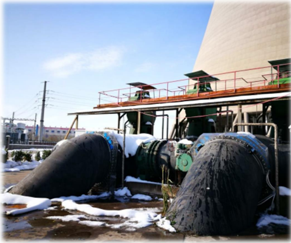
Circulating Cooling System in Power Plant using river water.
